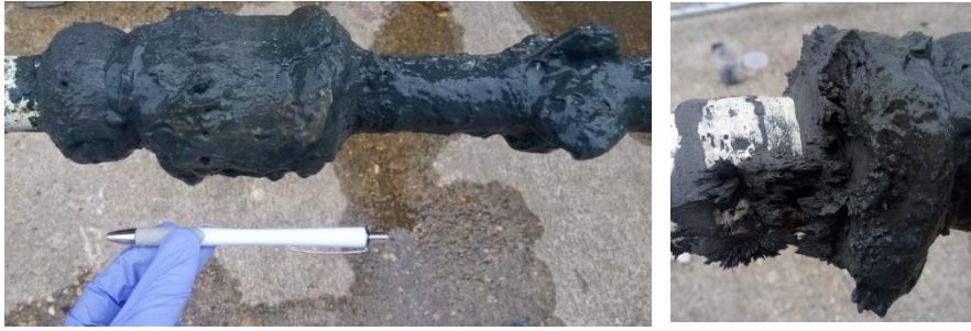
Fig. 29. CIP particle build-up in front of the permanent magnets
