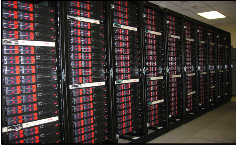
Figure 24. SuperMike-II supercomputer at LSU
