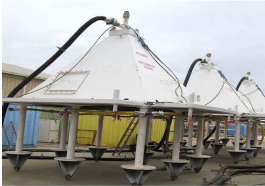
Figure 57: Cone shaped collector used in oil suction on Taylor Energy’s buried platform (from RRT-6)
