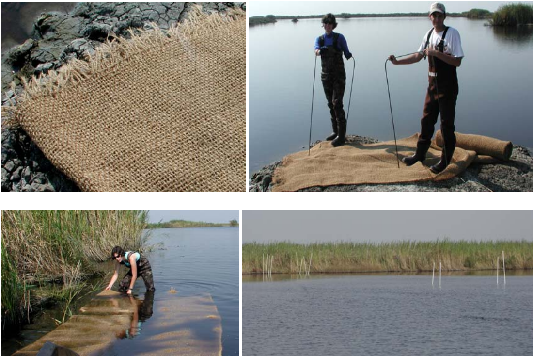
Figure 4. From top left, clockwise: (1) coconut mat texture before installation, (2) rebar and a coconut mat before installation, (3) coconut mat during installation, (4) white PVC poles mark the edges of the installed coconut mats.
