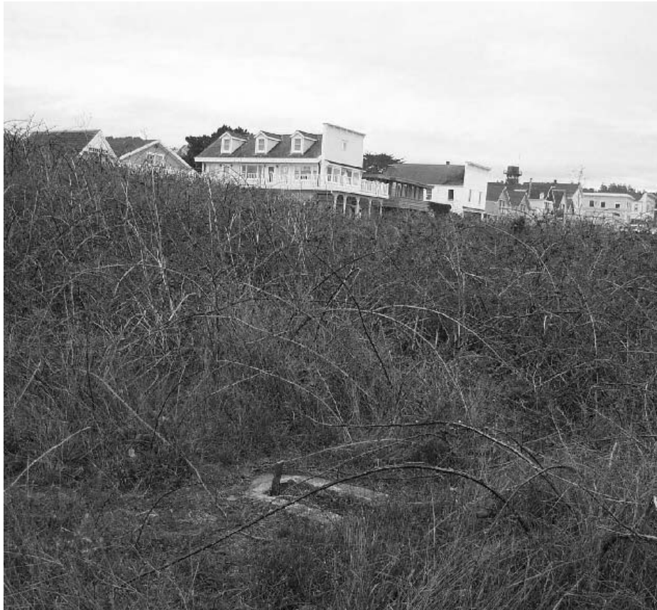
Figure 4 Footing obscured by vegetation near original mill.
