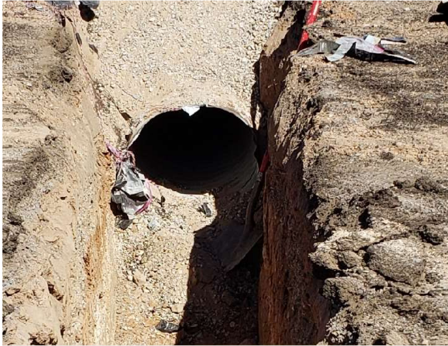
FIGURE 13 Buried corroded metal pipe
