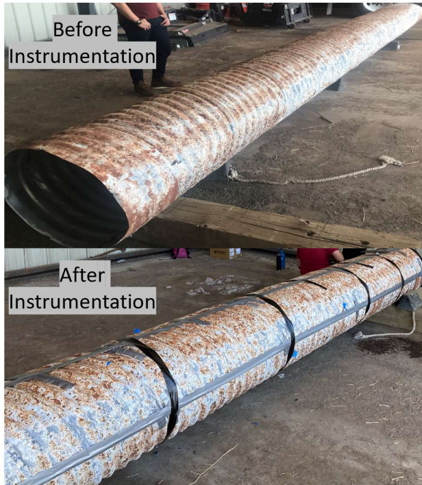
FIGURE 11 Corroded metal pipe before and after instrumentation
