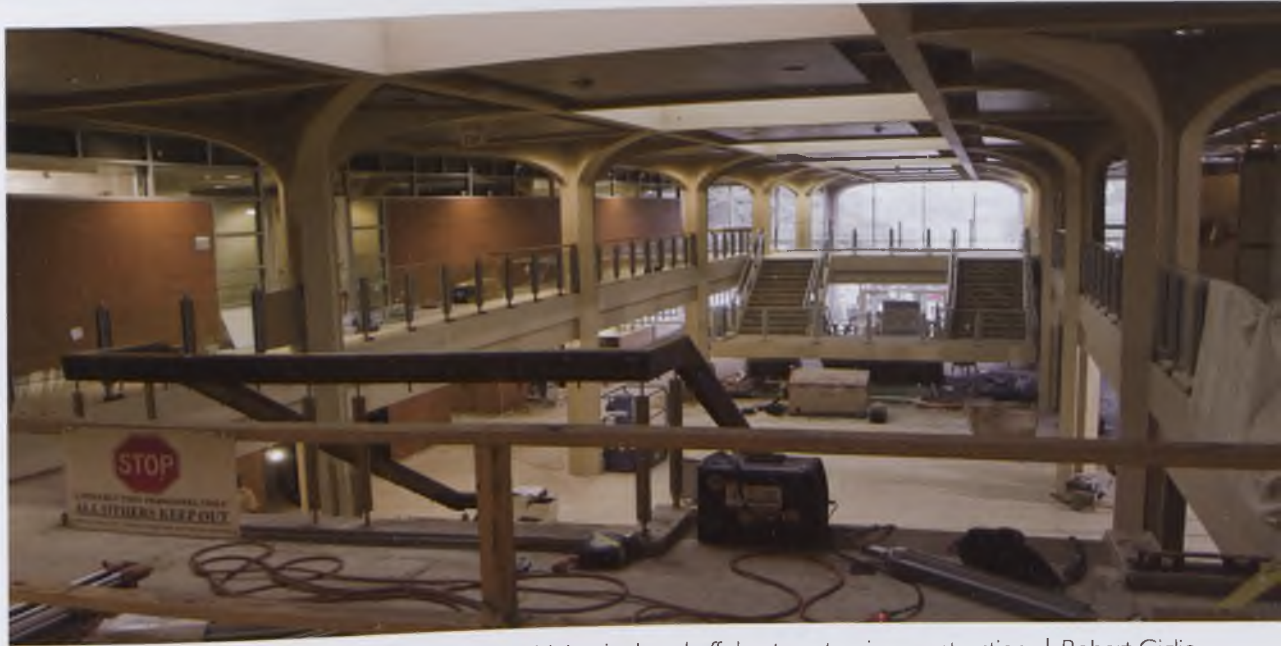
The front of the Union is closed off due to extensive construction. | Robert Giglio
