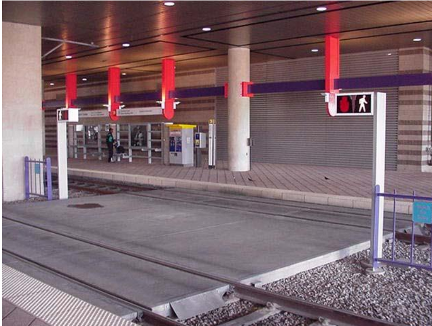
Figure 36. Pedestrian signals, DART, Dallas, TX
