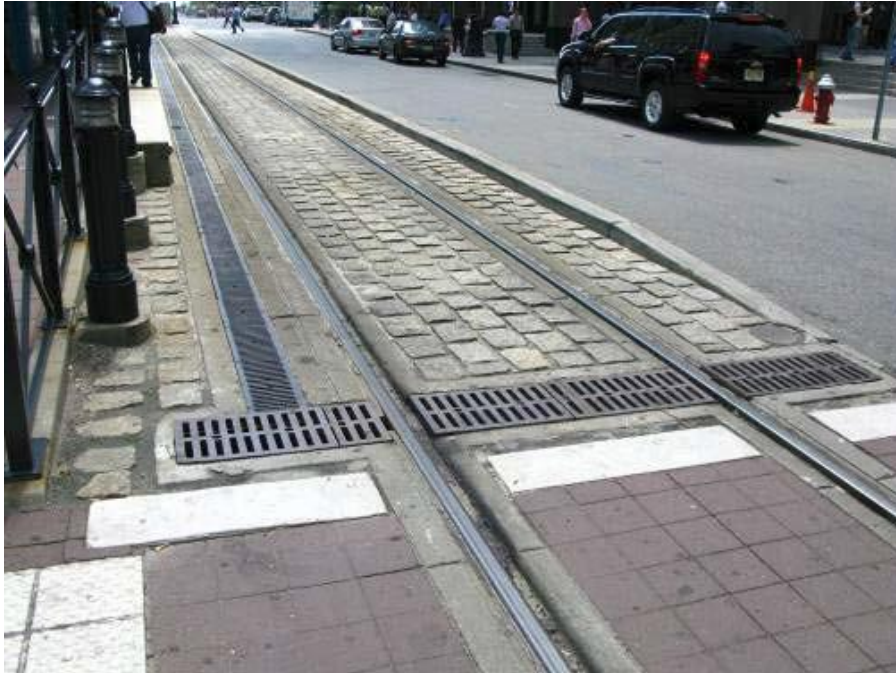
Figure 12. Type b.3 Alignment with Textured Surface and Drainage New Jersey Transit, NJ
