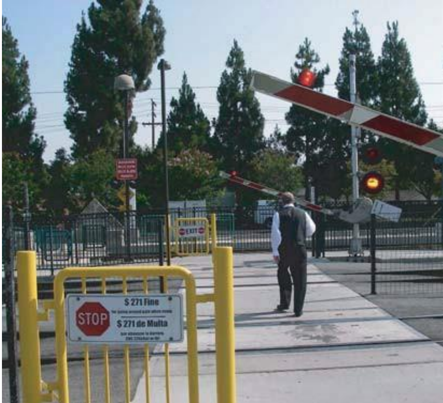
Figure 46. Pedestrian automatic gates in combination with pedestrian swing gates, Mountain View, CA
