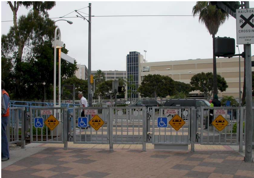
Figure 44. Pedestrian swing gates, Los Angeles, CA
