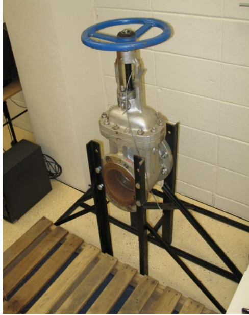
Figure 3: A 15 cm manual gate valve with a 36 cm diameter handwheel.
